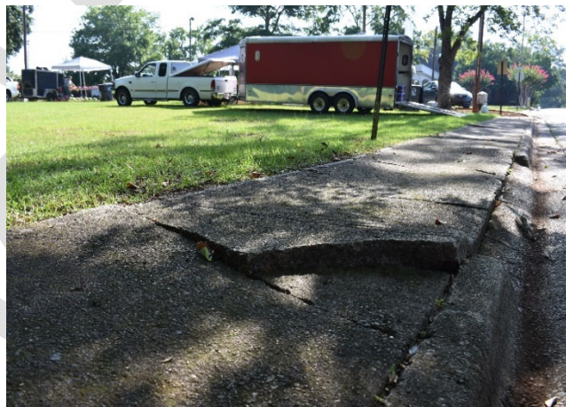
Picture 10: Cracked sidewalk in Forsyth
